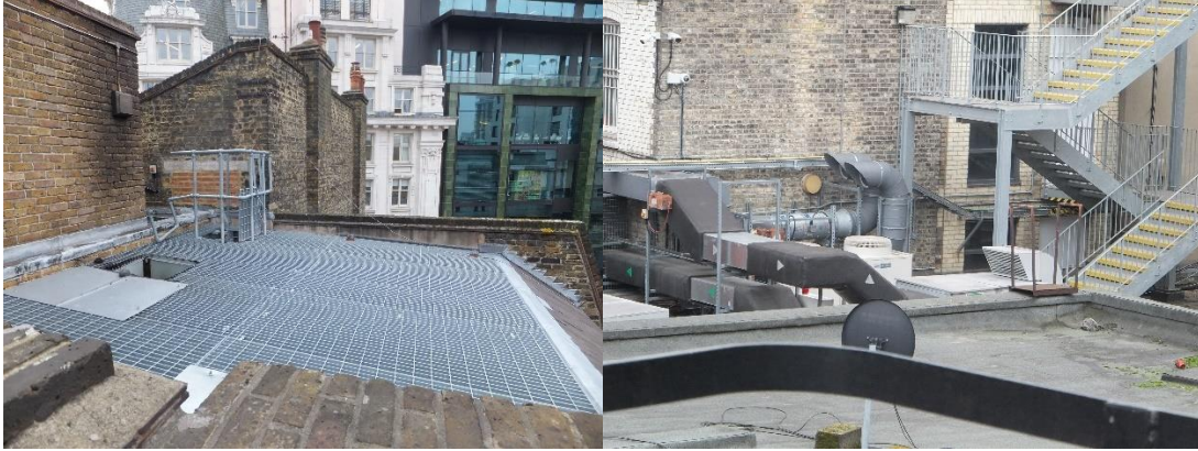
Figure 4 Photograph of plant room (left) and kitchen extract fan (right)
